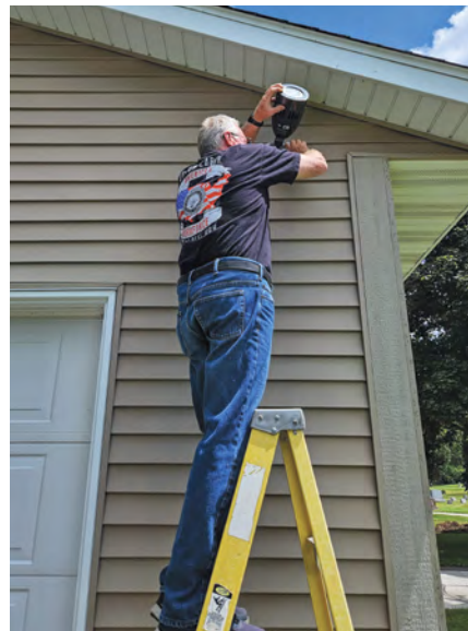
Retired Local 494 member Mike Zimmerman installing the flagpole light at Sheboygan Falls Cemetery.
